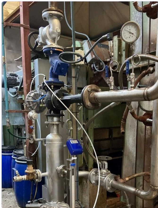
The recirculation station: the Jetomat with its actuator, above the separator and its level gauge.
