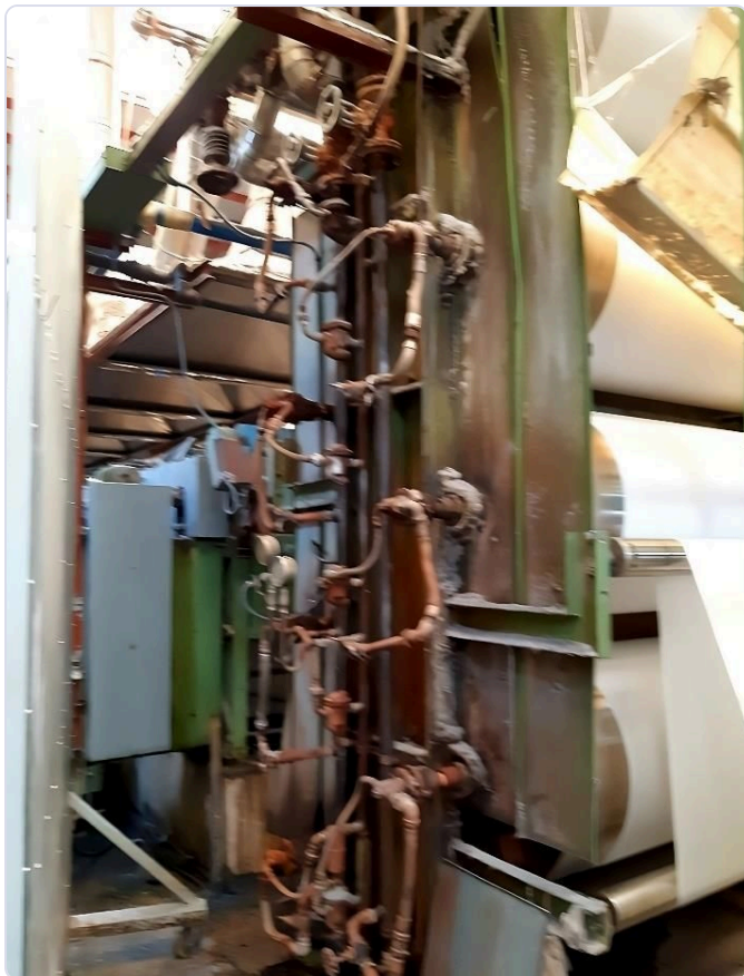
The tower of eight drying cylinders, with its steam and condensate piping.
